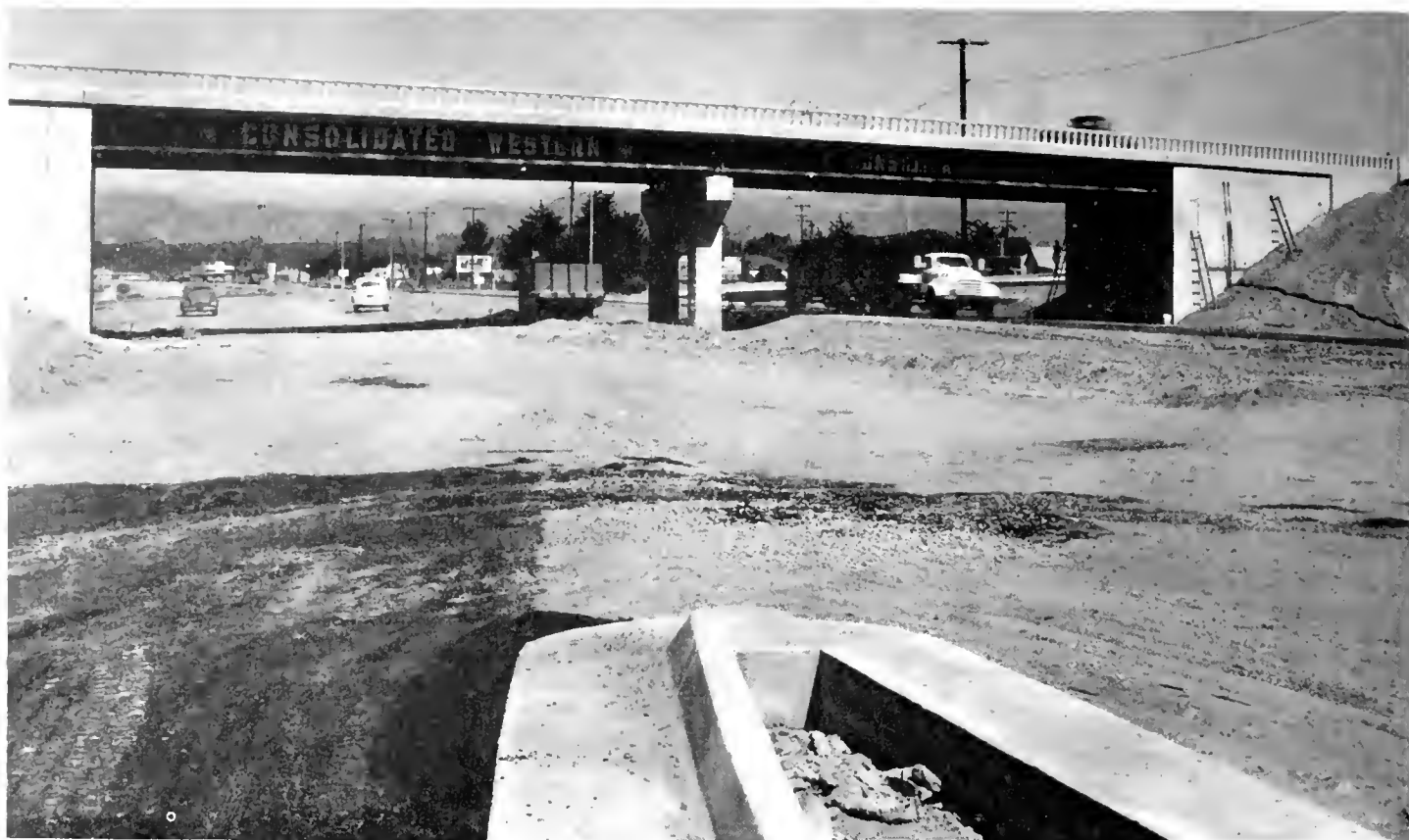
The mountains back of the City of Ventura are framed by the separation structure of the intersection with Saviers Road. Picture taken from southbound off-ramp prior to placement of untreated rock base and plant-mixed surfacing on southbound lanes. Pneumatic-tired compactor seen in center proved most effective in consolidating granular fills.
